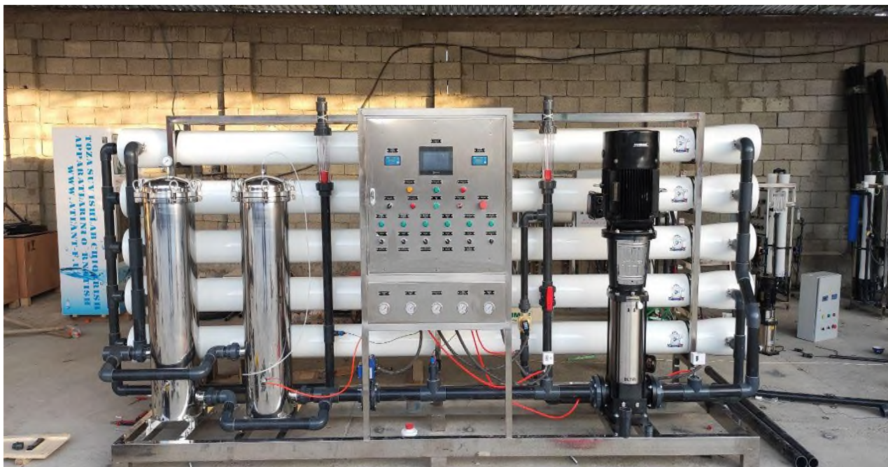
Figure 7. Rainwater filtration equipment
